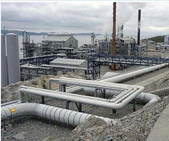
Power plant at Tjeldbergodden
